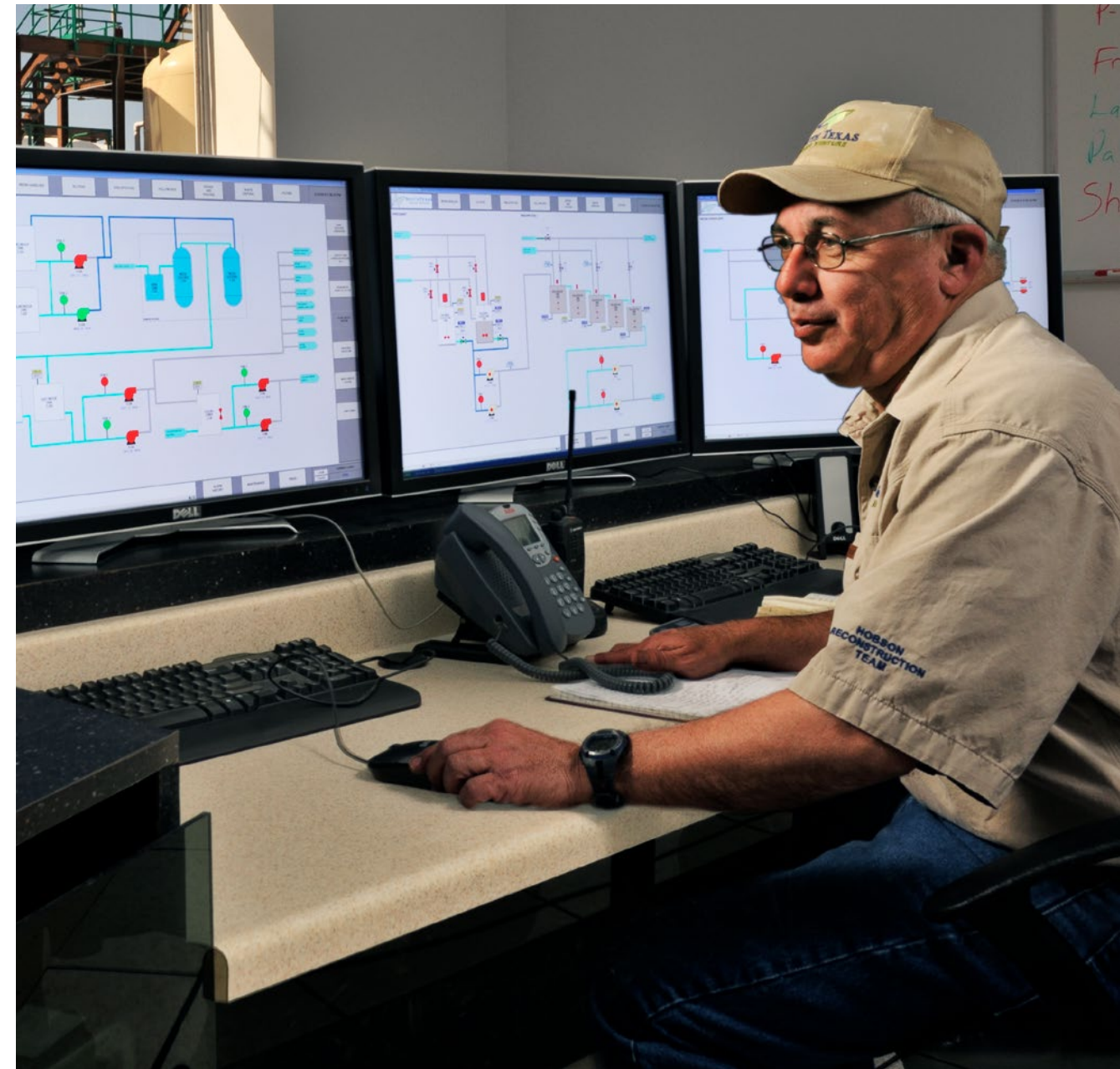
UEC Hobson control panel
